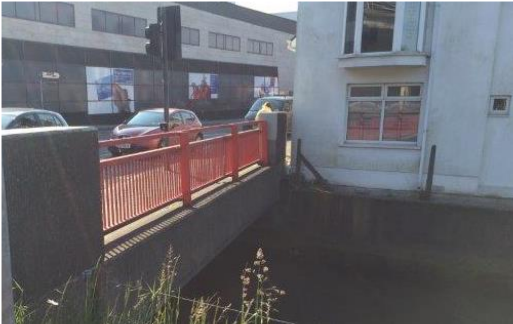
Figure 3.7: View of R851 bridge over the Tramore River and view of right bank. Note location of building directly on the river bank.
