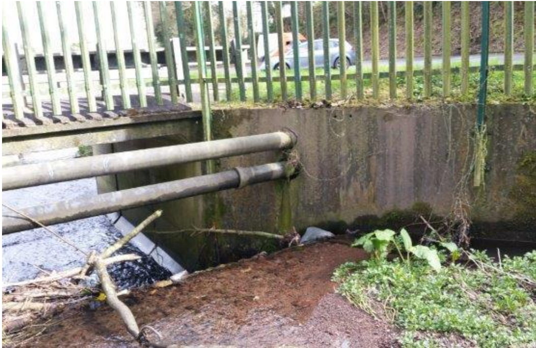
Figure 3.9: View of existing coarse trash screen at northern end of the Commercial Centre. There is a considerable difference in levels upstream and downstream of the screen
